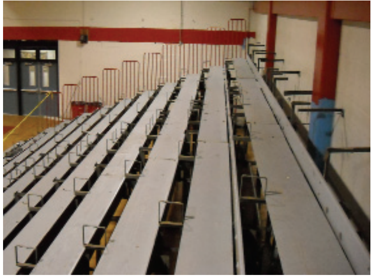
The existing footboards were replaced with code-compliant footboards. Existing heelboards were refinished in the same color as the footboards.
