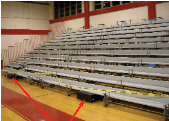
Sections were unanchored and re-aligned to eliminate gaps between sections. Motors were installed in conjunction with rigid row ties.
