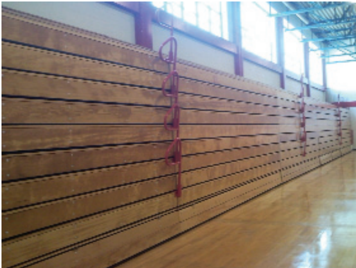
Fully refinished to "as new" condition with the Century Design no-sag system and with all safety equipment installed. Note the even row spacing across the entire bank.
