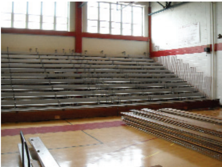
First step is to remove the fir lumber from the bleachers for refinishing at Bleacherman's facility. The understructure (manufactured by Wayne) was repaired and serviced.
