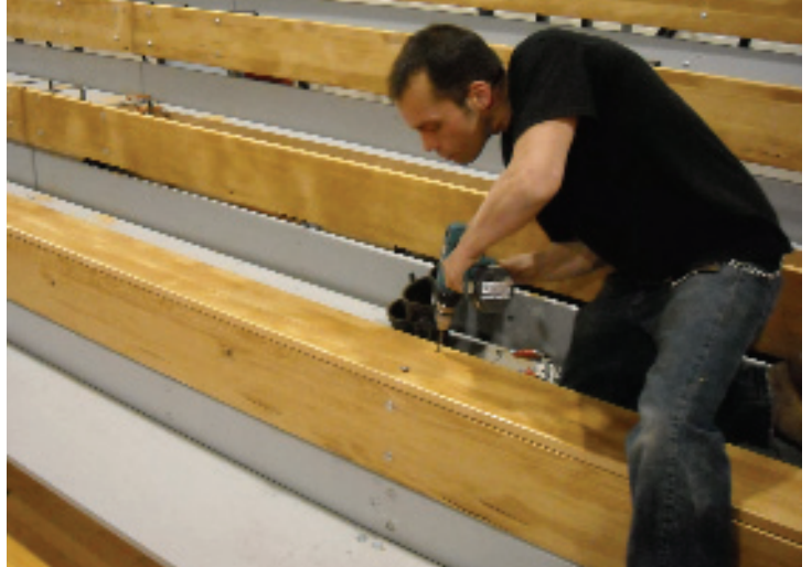
After being planed, edged, sanded and receiving three coats of approved sealer, seatboards and risers are reinstalled with new hardware
