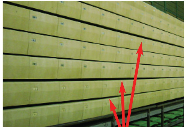
Bleachers sagging in the middle.
