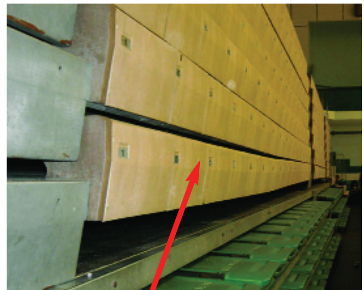
Another view of sagging at the end of the bleacher section.
