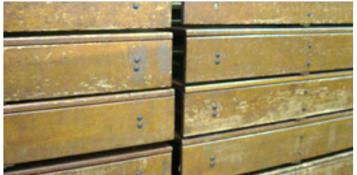
The wood bleachers in the Chase Gymnasium showed their age. Note the gap between sections.
