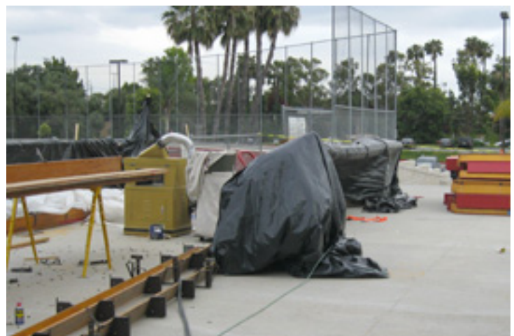
Bleacherman's sanding/edging/refinishing equipment set up outside at Biola University. Seatboards and risers were recycled and refinished on-site.
