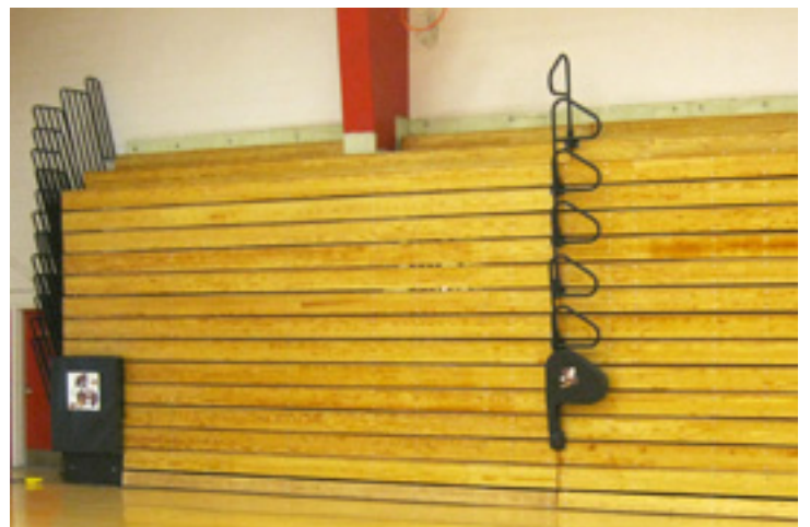
Refurbished Bleachers in closed position. Note padding on ADA rail at end, also customized with the school mascot.
