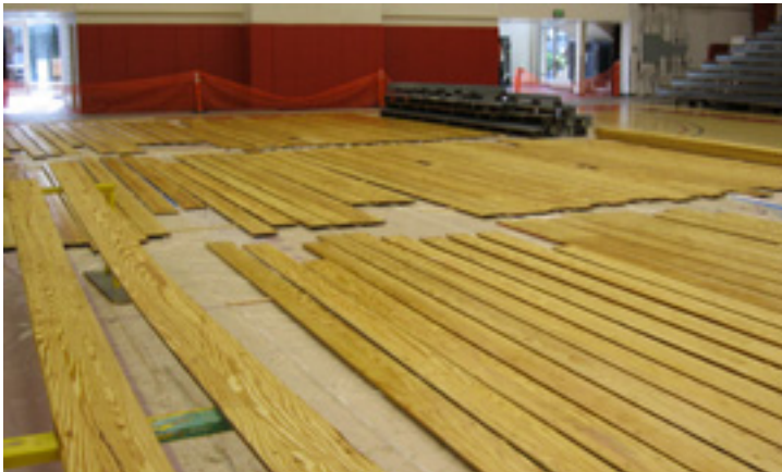
Floor is protected with plastic, when refinished wood is brought back into the gym for reinstallation.
