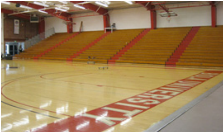
Outdated bleachers lacked proper safety equipment required to be code-compliant. Other serious problems are hidden from view, underneath the bleachers.
