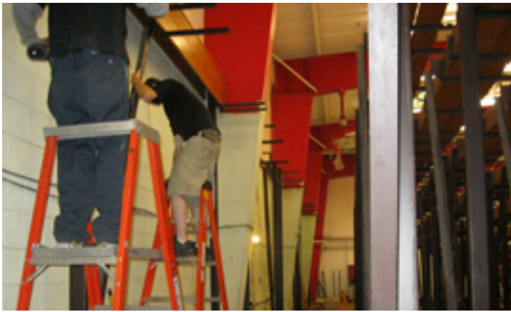
First, the Bleacherman crew unbolted the old bleachers from the wall, in order to join the sections together flush and remove the top row.
