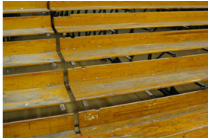
Seat boards and risers are removed for planing and edging. Heelboards and footboard remain in place for refinishing.
