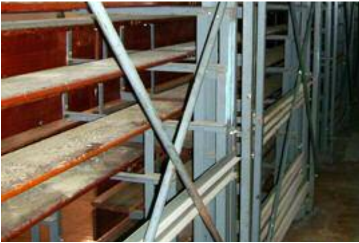
View from the back. Floorboards are extensively worn. Most of the understructure was sound, with minor rust, mainly on the lower portions.
