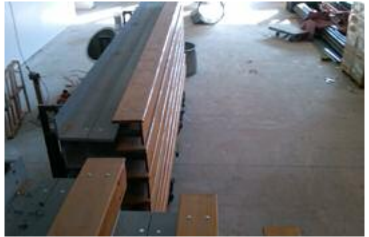
Reconditioned bleachers are ready to be re-anchored in the next step of renovation.
