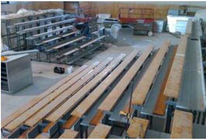
All of the bleachers were unanchored from the wall and moved, so that floor renovations could proceed. Note new riser boards on floorboards, “staged” for installation.
