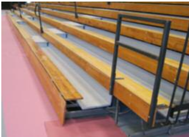
Bleachers are nearing completion, with P-rails, intermediate steps and ADA cutouts installed.
