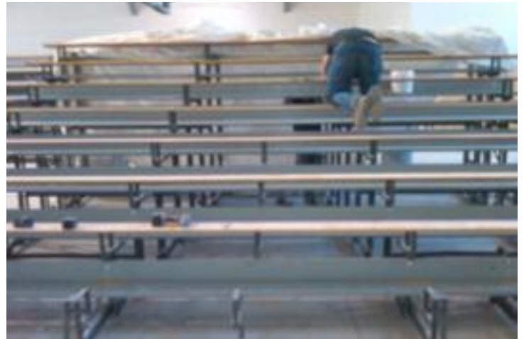
Bleacherman crew members are beginning to re-attach refined lumber. Floorboards and heelboards have been primed.
