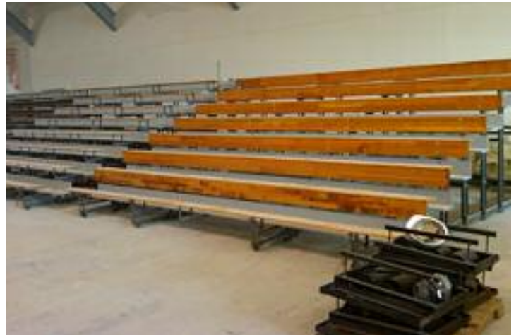
Work in progress: the bleacher section in front has new seats and risers installed.
