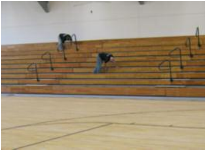
Applying the final seal coat. Owner was very particular about appearance of the refinished bleachers.
