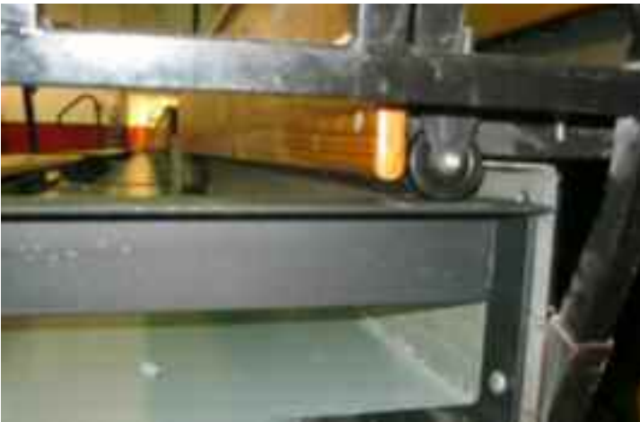
Sagging of bleachers (which makes them hard to open and close) is prevented with the addition of the patented Century Design® “no-sag” system, after the understructure was repaired. This photo shows a Century Design® wheel on a seat-level runner at the end of the bleachers.
