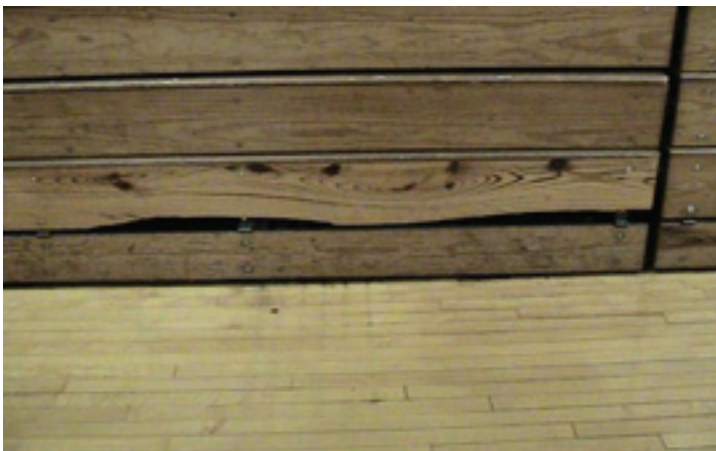
An original Southern Yellow Pine board was replaced with a locally-sourced Pine board with lots of knots. It has broken at the bottom and should be replaced.
