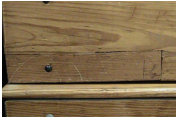
Here's another attempted repair, where a chunk of wood was bolted in, to replace a broken piece.
