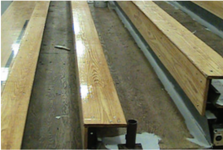
Plywood deck system was unsightly and needed to be finished for an as-new look. Photo above shows the footboards prepared for painting -- workers have started edging the heelboards prior to painting the deck.
