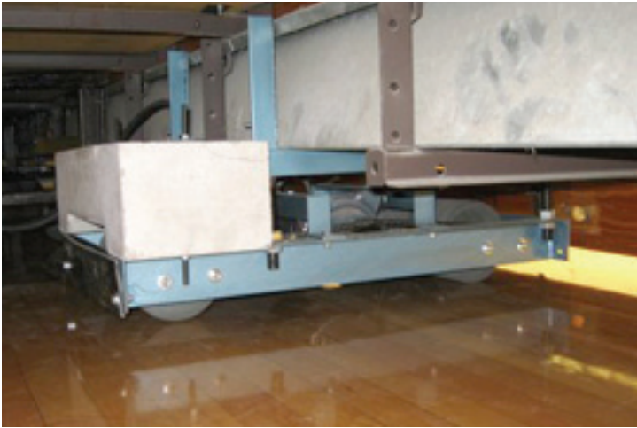
New motor drives were installed by the previous contractor. Even though these are brand-new, the motor drives were not working properly. Note white concrete weight mounted on the back of motor drive.
