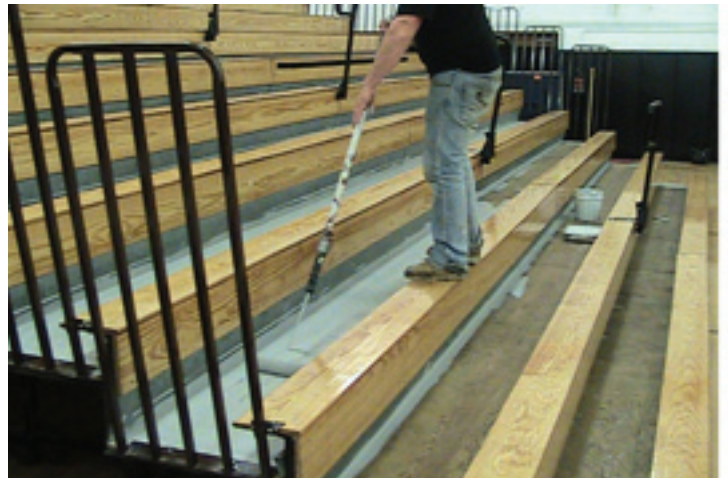
Here the worker is applying the first of two coats of approved deck sealer. The contrasting color is required by ADA, for those who are color blind or have depth perception issues.
