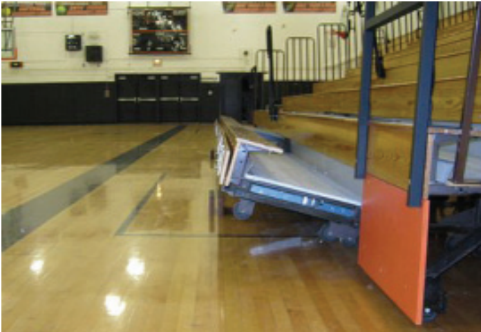
During operation to full open position, the first row would tilt up -- the front wheels of the motor drive and the bleachers would lift up, damaging the first row.
