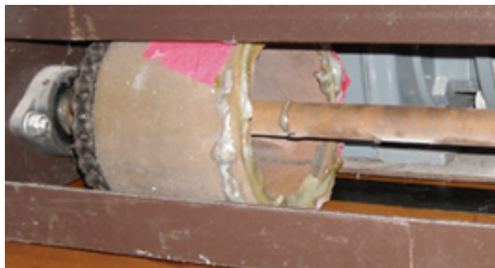
Delaminating drive roller in a drive unit.
