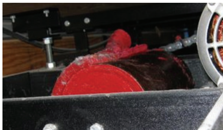
This drive roller shows how the urethane covering is peeling away from the drive roller.
