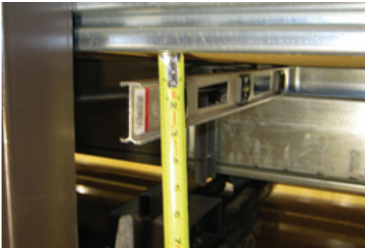
Carpenter's level shows that the footboard is sagging (even in the partial open position) approximately 1 inch toward the front of the bleachers. In the closed position, this row sagged approximately 3 inches.
