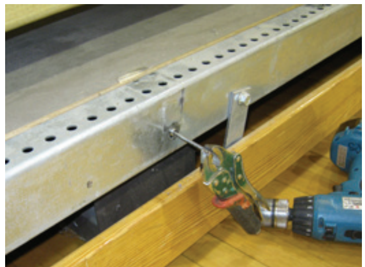
The bolt that held the seat bracket to the nosebeam was sheared off by the sagging row above. Here, the broken bolt is being removed (with an Easy-Out) for replacement.
