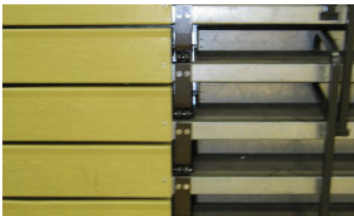
This photo shows the foot level Century Design® at the aisles in the closed position. (Note the even row spacing, now that the bleachers have been repaired to as-new condition.) Even if climbing does occur in the closed position, Century Design® guarantees that the rows cannot sag.
