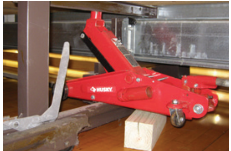
The first step is to straighten the understructure. Here a large floor jack is used to lift the bent arm to the correct position.
