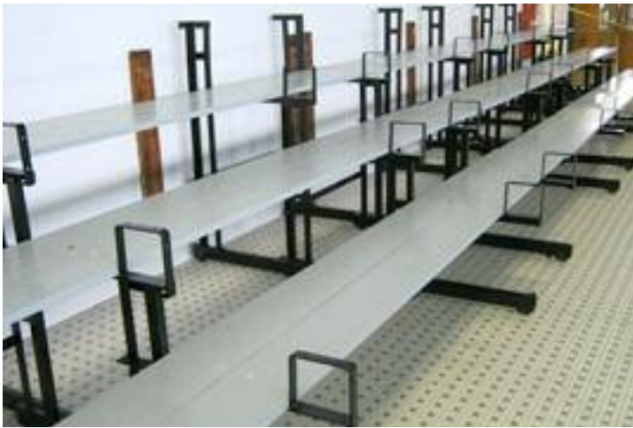
Footboards go on first, as the new bleachers are installed. Heelboards will be attached next. Bleachers are being made code-compliant, meeting closed-deck safety requirements.
