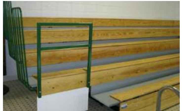
ADA cut-out for wheelchair with safety rail and self-storing end safety rails installed. Like the P-rails, they match the school's colors. All painted surfaces received multiple coats of marine-grade coatings to resist moisture.
