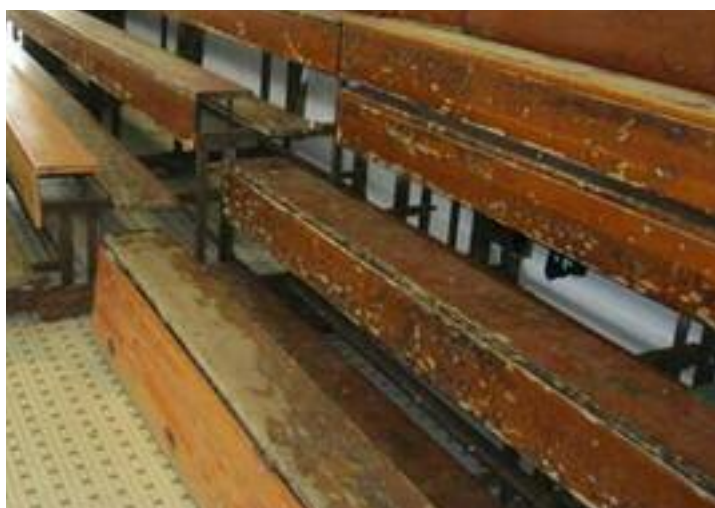
Bleachers on both sides of the natatorium were affected. The finish on the wood is completely discolored and worn away in some areas.
