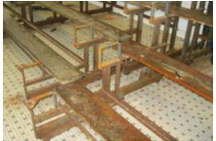
Some of the bolts were so rusted, they had to be cut off in order to remove the wood.
