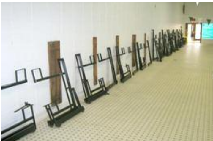
Original understructure (after remanufacturing) is “staged” in position before anchoring to the wall. Note floor has been cleaned before understructure is re-installed.
