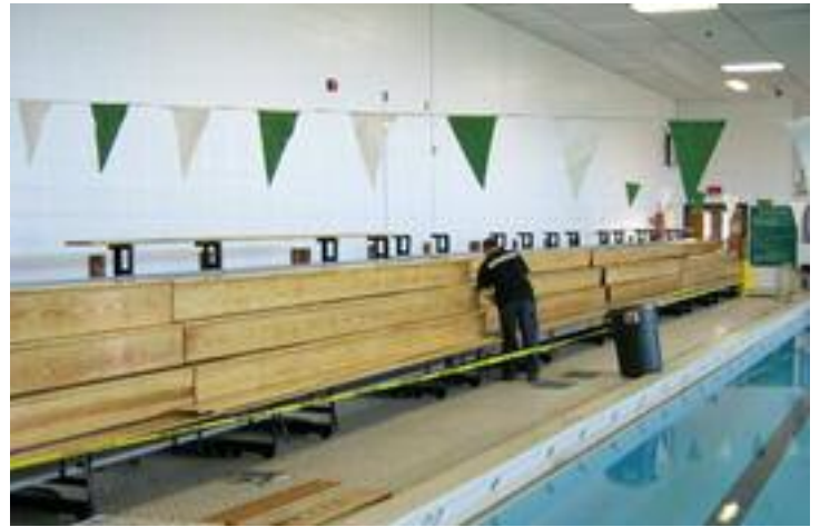
Reconditioned Fir wood seats and risers are installed. It's hard to believe this is the same wood that was removed from the original bleachers. They look new again!
