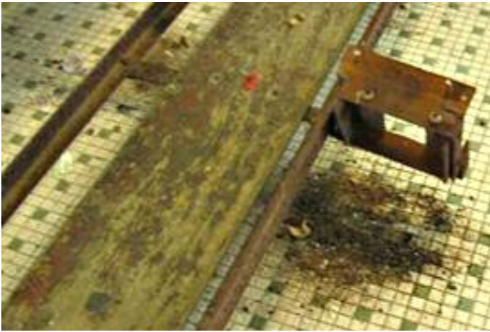
Lumber is removed for refinishing, as the first step in dismantling the original bleachers.
