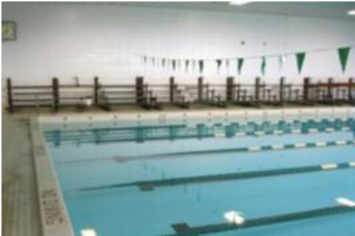
Most of the boards have been removed in this picture. Lumber was recycled for use in the new “closed deck” bleachers. The original understructure was salvaged and rebuilt at the Evergreen manufacturing facility.
