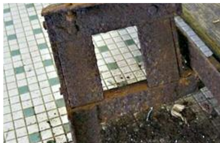
When the Bleacherman started to remove the wood, what we found was even worse - a badly corroded understructure on the first row only. The first row understructure was remanufactured - fabricated by the Bleacherman.
