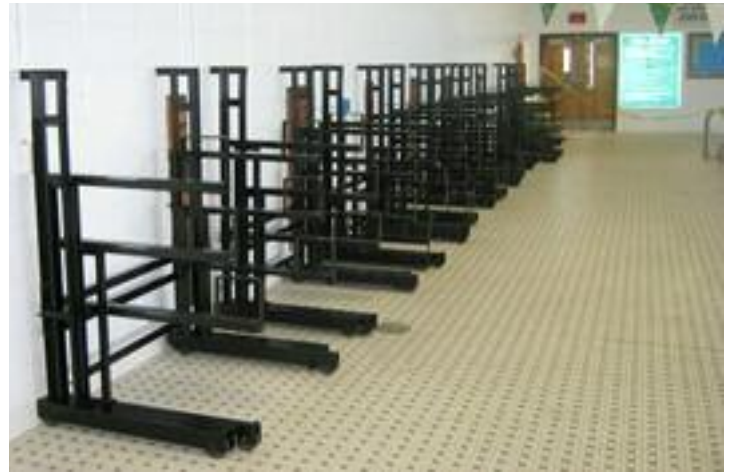
Evergreen Bleacher understructure now anchored to wall. This understructure has been sandblasted, powder coated with special baked-on rust-resistant paint, then powder coated again.
