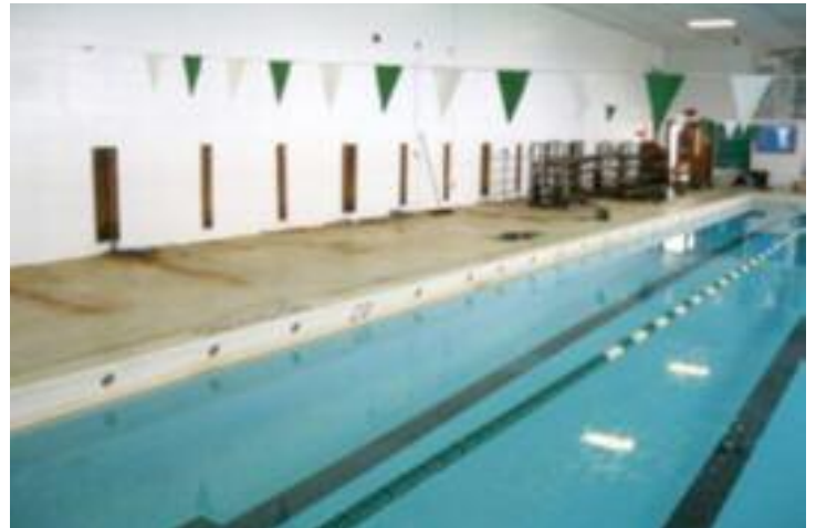
The Bleacherman crew has one more section of bleachers left to remove in this photo. Note staining of floor below where the bleachers used to be located.
