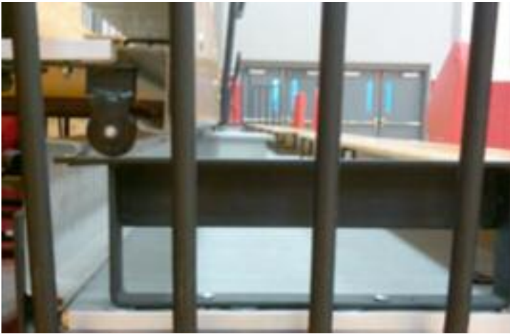
Close up of Century Design® wheel on runner in the full open position. These bleachers were required to meet a “no-sag” specification in the bid.
