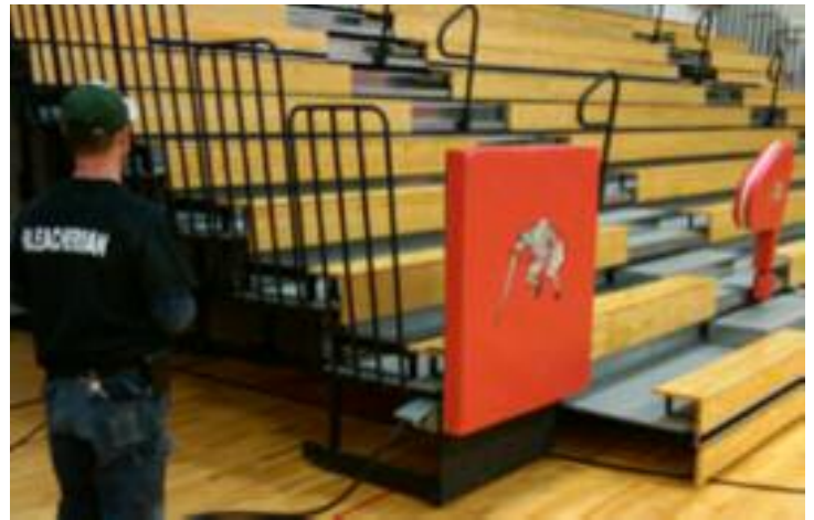
Self-storing safety rails and P-rails remain in position at all times, unlike the original bleachers. This provides an extra measure of safety, beyond the minimum code requirements and gives added consideration to those in wheelchairs.
