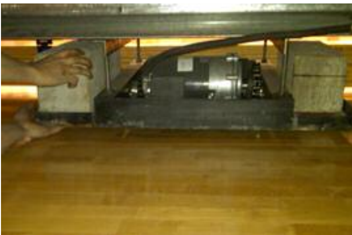
Installing the ballast blocks on the heavy-duty motorized drive underneath the bleachers. The motors are 110 volt, allowing the extra safety option of “no live wiring” underneath the bleachers.
