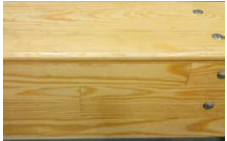
New seats are solid Southern Yellow Pine. The riser below is the original laminated board that was recycled from the old bleachers. The recycled laminated boards were planed, edged and sanded to match the new seats. With new hardware, everything looks new!
