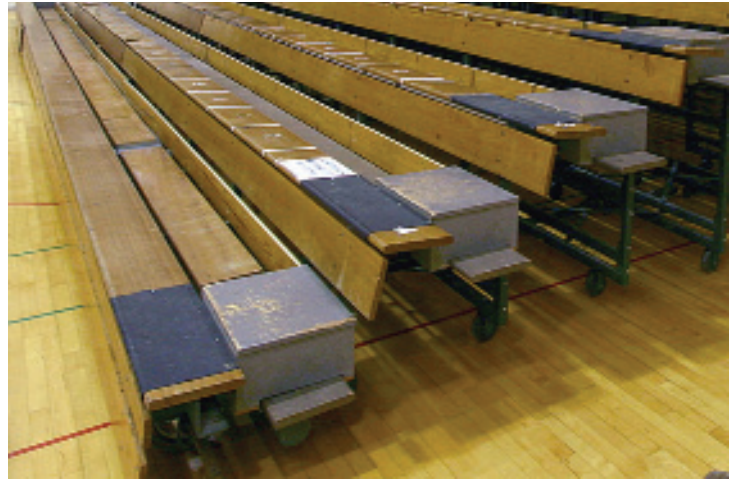
"Homemade" seat-level aisles were added by the owner, in an attempt to improve ingress/egress.
