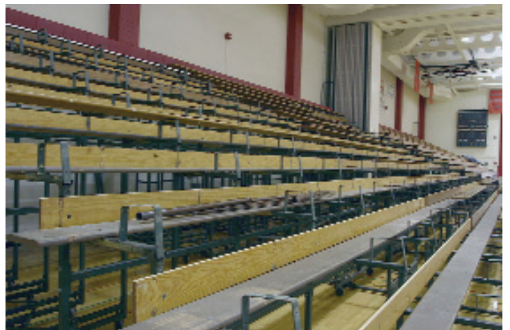
Removal of the seatboards and risers in preparation for the installation of the plastic seat modules.
