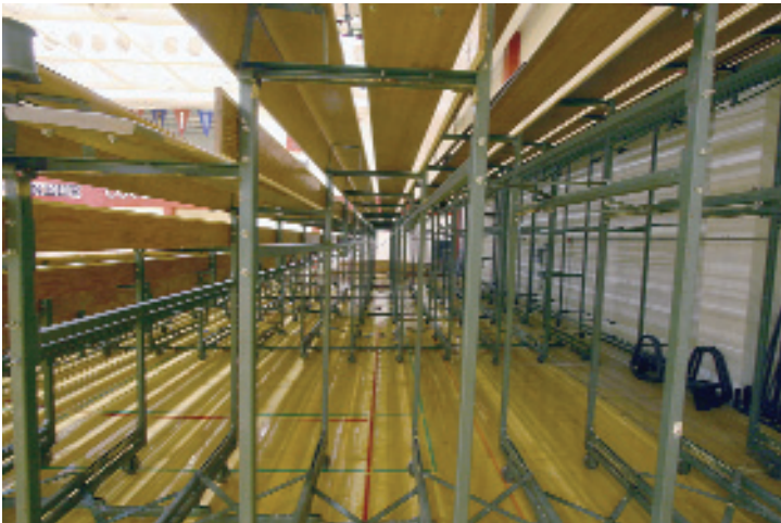
Original understructure needed minor repair and service but was otherwise in good shape. Berlin understructures have a unique adjusting system, not available in new bleachers.
