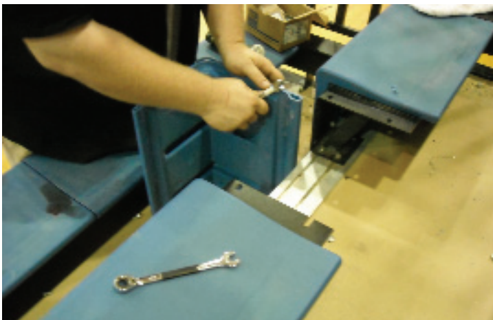
Plastic seat modules that are obtained from the "American Flag" section are used to replace deformed or damaged ones. Here a seat is being trimmed to size before mounting.
