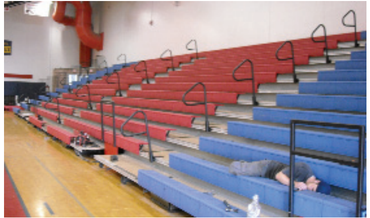
Seat modules are being installed. Most of the safety equipment is in place, while additional ADA wheelchair cut-outs are in progress.
