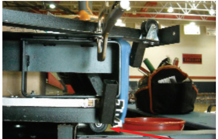
After the sagging understructure is corrected, the Century Design® no-sag system is installed. Note the wheel resting on the runner. This raises the row to the correct position.
