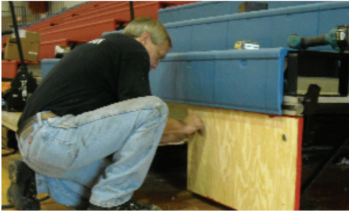
Installing ADA wheelchair space. ADA safety rail will be mounted here in compliance with ADA requirements.
