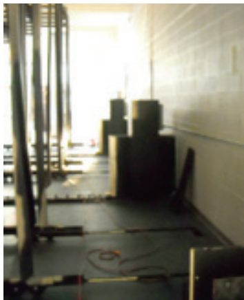
Five motors drive units that work together to open and close the bleachers.
