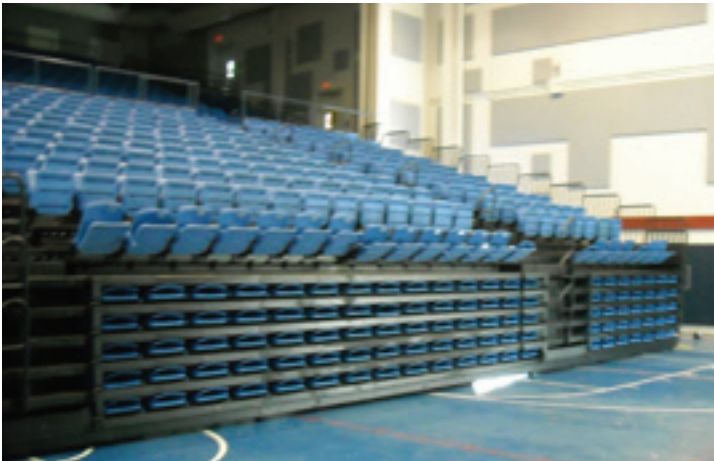
Because the platforms were sagging, they were difficult to close. A scraping/grinding noise could be heard when the folding platforms were operated.
