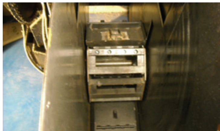
The metal chain links are taken up on sprockets in the motor drive unit as the platforms are retracted to the closed position. These reverse fold metal links are 10.325 inches wide, but even these very heavy-duty links can be severely damaged when the platforms sag.
