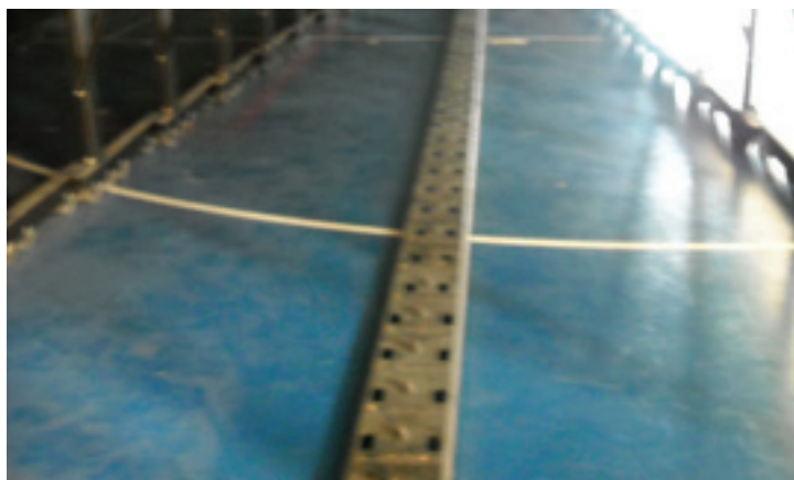
The metal chain links lay flat on the floor, when extended to the full open position. Seen here after repair and replacement of broken components. Platforms and their motor systems are specially built, very expensive to repair. That's why it is critical to install a Century Design® no-sag system -- to prevent future sagging and redundant, expensive repairs.
