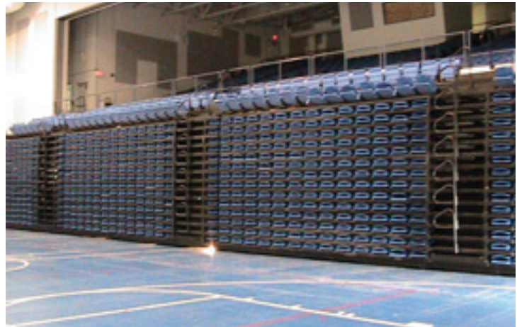
Because of damage incurred during opening/closing, the platforms would not retract completely and intruded upon the space needed for gym activities.
