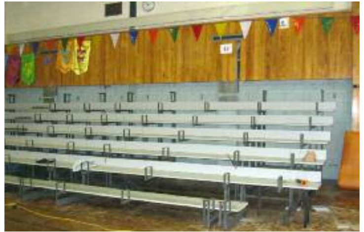
After footboards are attached, heelboards are installed. The new bleachers will have a “closed deck” design, with no gaps that can present a safety hazard.
