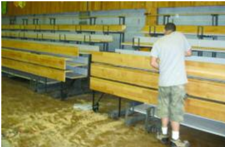
Bleacherman crew member installing newly refinished risers and seats. All the original Fir lumber was reused, for a fraction of the cost of new lumber.
