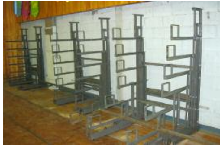
Evergreen Bleachers™ understructure being installed. Owner wanted to continue with a “four-horse” system for durability and longevity.
