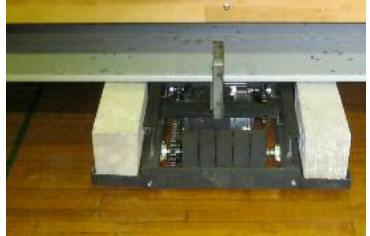
New motorized drive with ballast blocks on each side is attached at row one. New bleachers will open at the touch of a button, instead of being manually operated.
