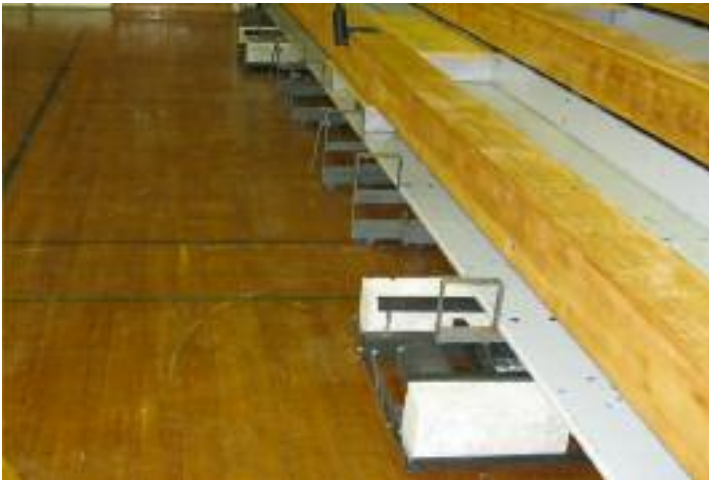
Two motorized drives can be seen on this bank of bleachers. The nosebeam and first row seats will be attached later.
