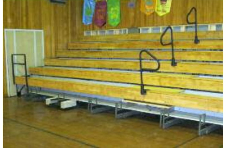
P-rails and ADA rails are installed. First row seat boards and noseboards are yet to be installed in this photo.
