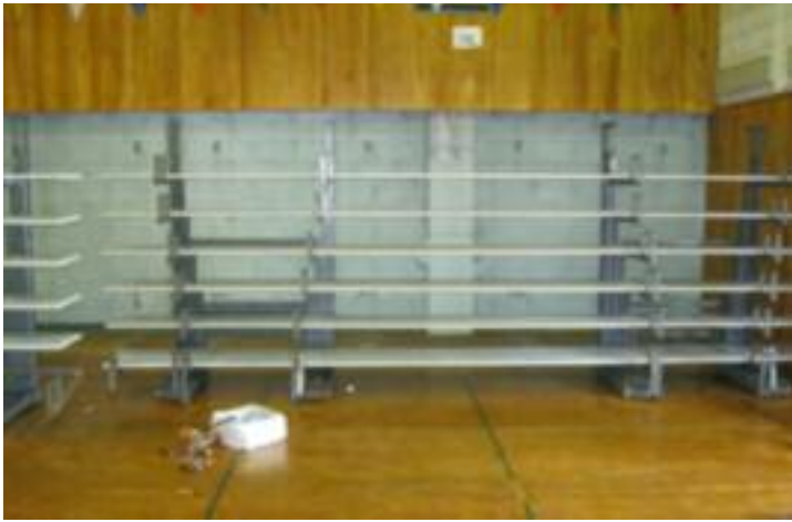
After the understructure was anchored to the wall, new footboards (painted gray) are installed.
