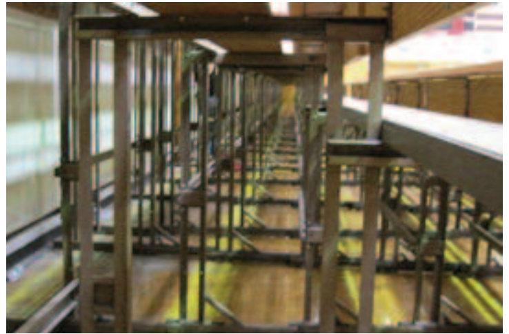
Another view of the understructure from below. The original four horse system (uprights) is much stronger than the two horse system of many new telescopic bleachers being sold today. Believe it or not -- these "low-bid" bleachers can span up to 26 feet with just two uprights!
