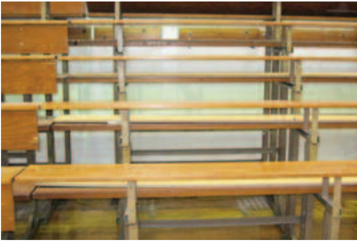
As risers and footboards are removed, the original "four horse" system of vertical support columns is exposed.
