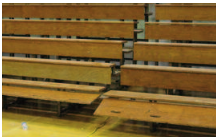
Many of the original riser boards had been damaged or broken, and were replaced by non-matching wood, as seen above.
