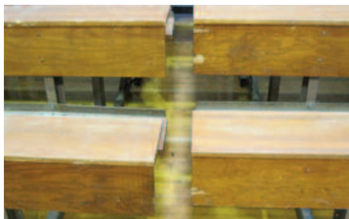
The original bleachers had large gaps between sections – a potential safety hazard. Note plywood replacement risers.
