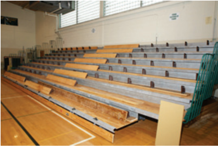
One bank of the Evergreen bleacher system is put into position, then new safety rails were installed, before the refinished lumber is refitted.
