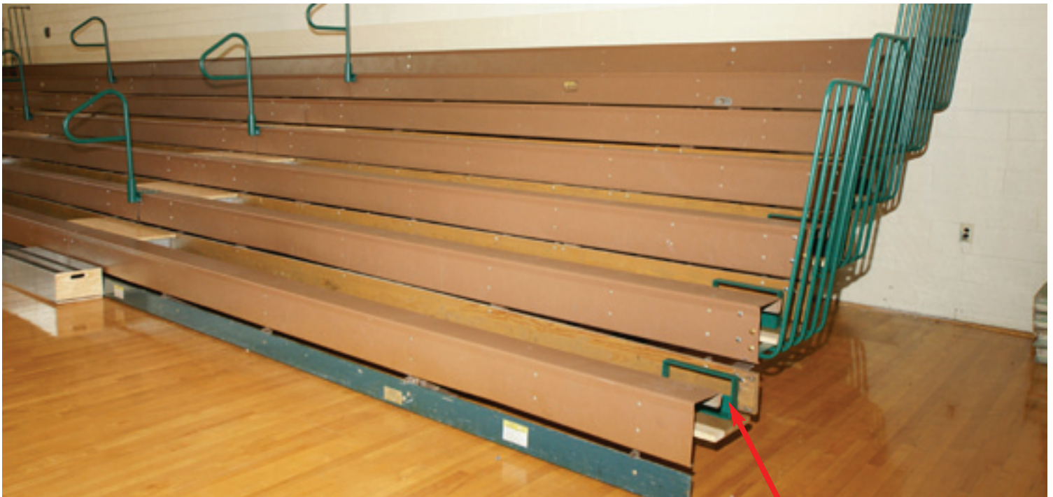
Vinyl on steel Interkal understructure was repaired to OEM condition, then outfitted with safety equipment such as P-rails, end rails and seat level aisles. All this is done prior to the Century Design® system installation.
