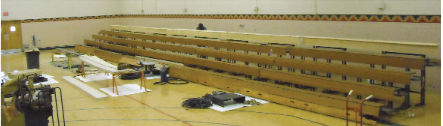
Original Medart bleachers were unanchored from the wall and moved forward, allowing room to repair the floor and wall behind bleachers. These bleachers had a lot of damaged wood, so top row seats and risers were replaced with new lumber.
