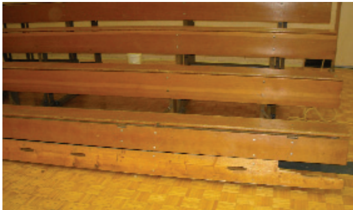
“Open deck” feature of original bleachers can be seen here. Because of the potential safety hazard, open deck seating will not meet most current code requirements.
