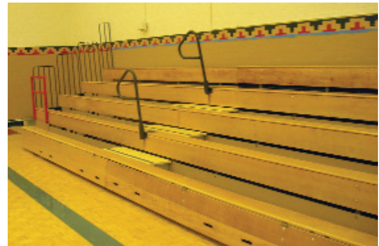
View showing intermediate aisles, P-rails, and self-storing safety rails on the end.
