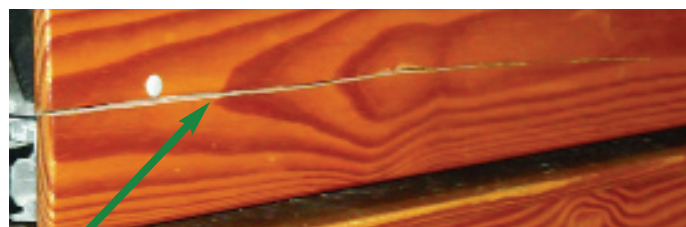
Cracked riser board in wood bleachers is an example of the damage to be recorded on the form.
